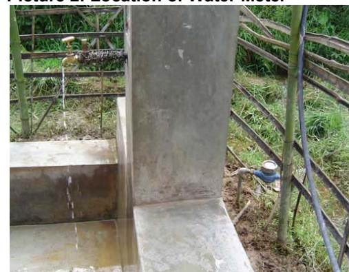
Picture 2: Location of Water Meter
