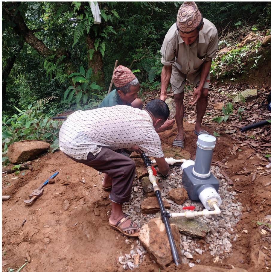
Installation of inline chlorination system
