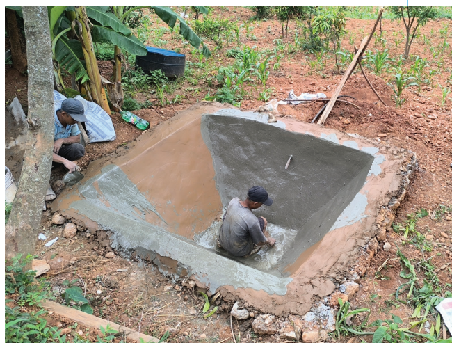
Construction of soil cement tank at Kangsang WASH project, Fikkal Rural Municipality-4, Sindhuli
