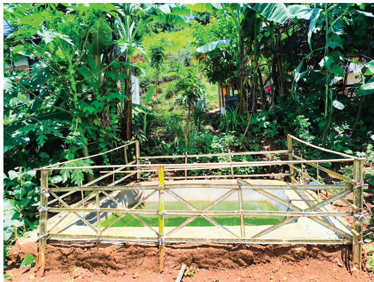
Soil cement tank to promote Multiple Uses of Water System at Chure Lamidamar WASH project
