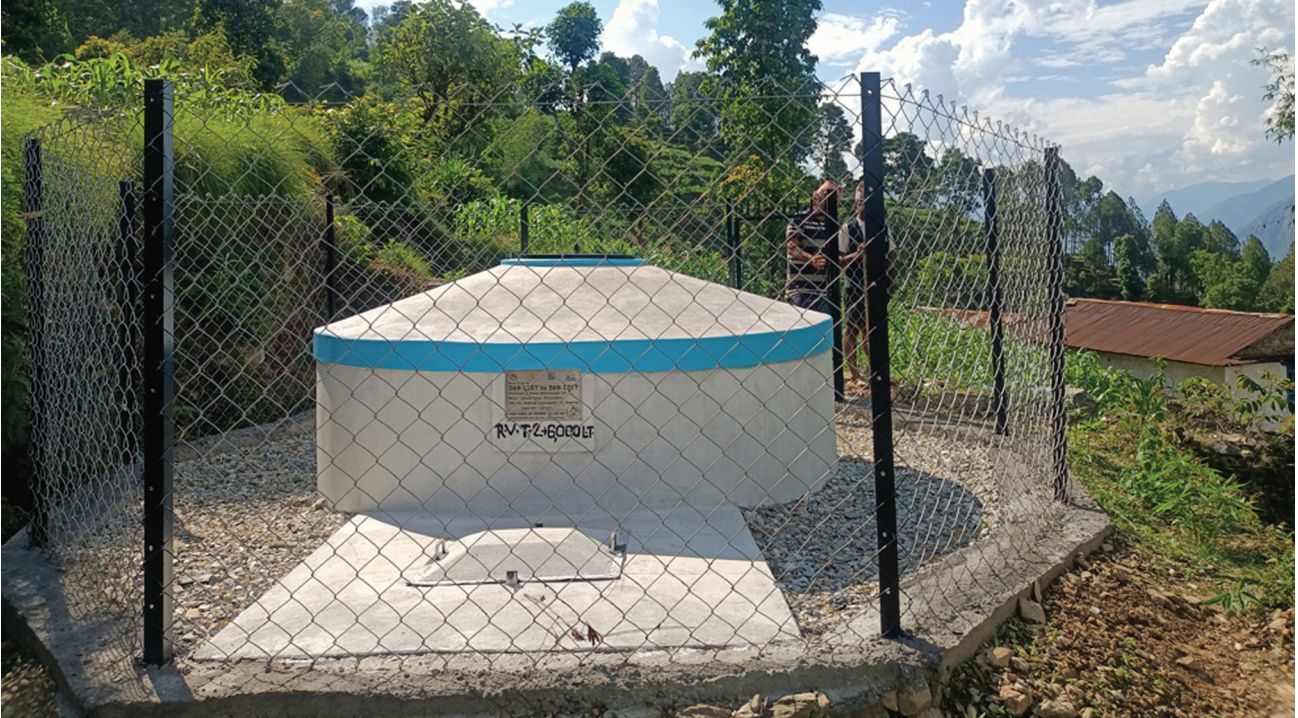
Reservoir tank at Kavredanda Lift WASH Project, Baglung Municipality-13
