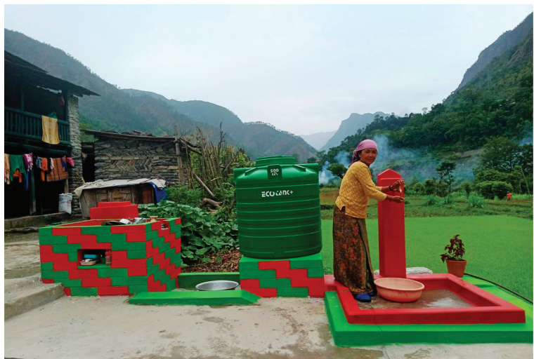
Washing Slab and Tap at household premises at Pakhu Kurshimla WASH Project, Mangala Rural Municipality-5
